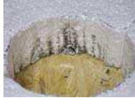
Fig. 8. Side wall of the collector C07 ring with vertical chains of holes.
