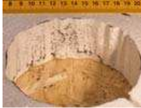
Fig. 7. Side wall of the collector C01 ring with vertical chains of holes
